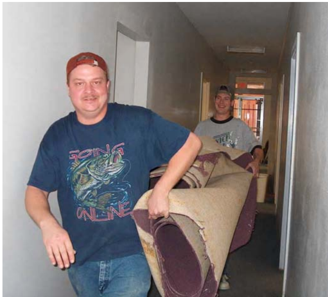
Ron Fry, Jr., left, and Jason Deevers pull up and haul out the damaged carpet throughout the building.
