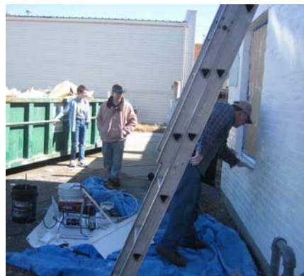
Members of the Greenville Home Church gives the outside of the building a fresh coat of paint.
