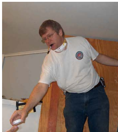
Brent Johnson from Aldersgate Church headed up the installation of all the wiring for our phones, computers and networking.
